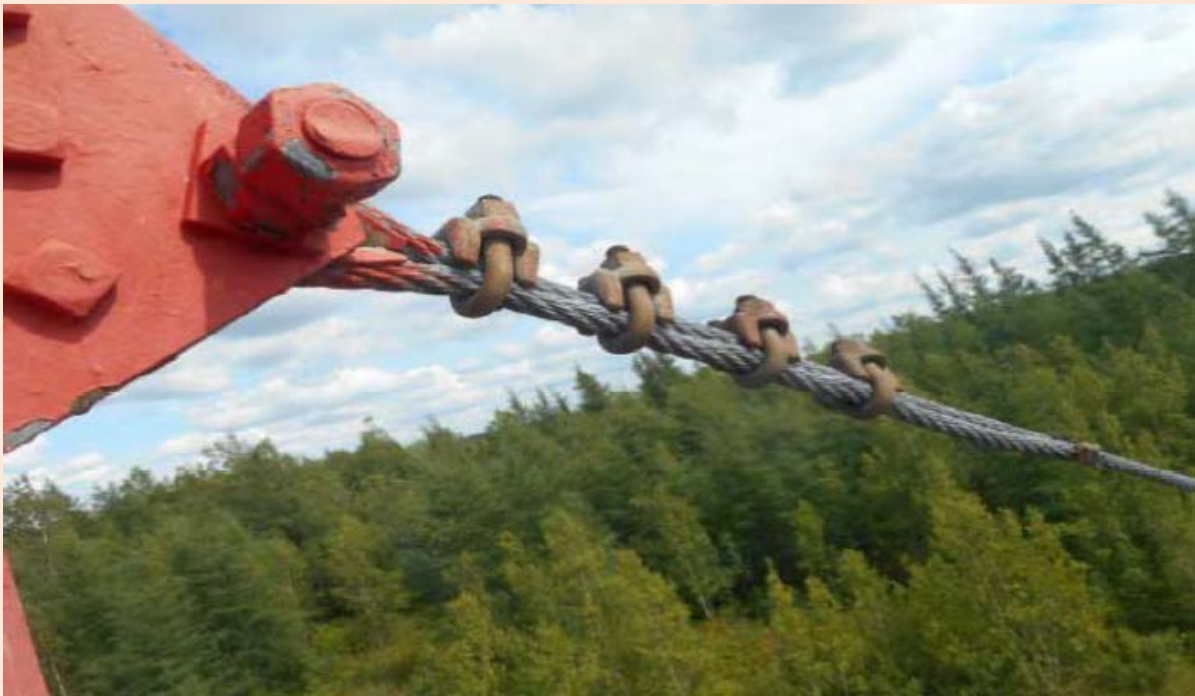
Wire rope guy termination at the tower end
