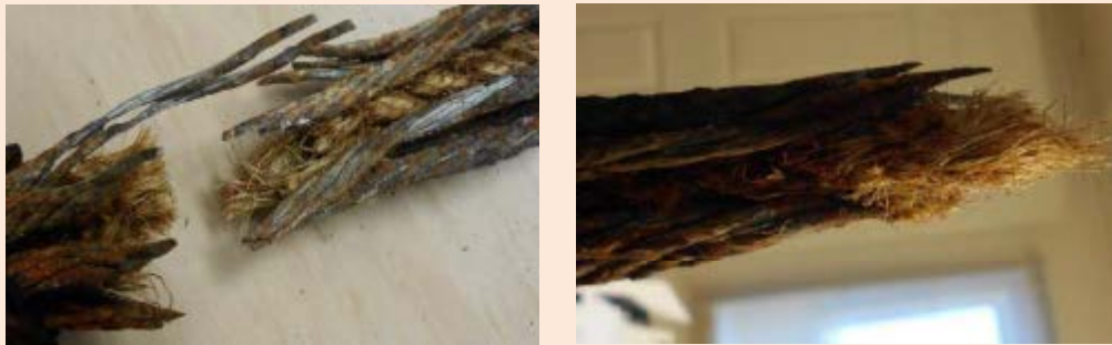
Severely corroded and broken wire rope fibre core guy
